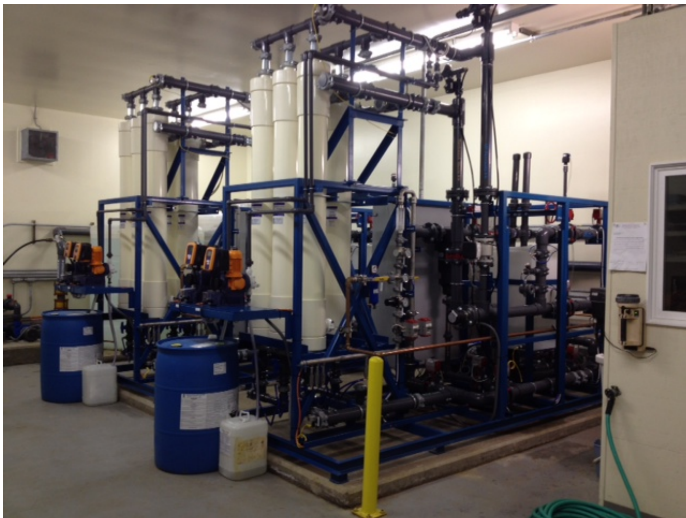
Water Plant Membrane Skids
